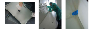
Fig. 3. Spots contaminated by DLST 1-18 isolate in the two hydrotherapy rooms: floor traps, wet surface under shower mattress and plastic rubber in a damaged corner of the mattress.
